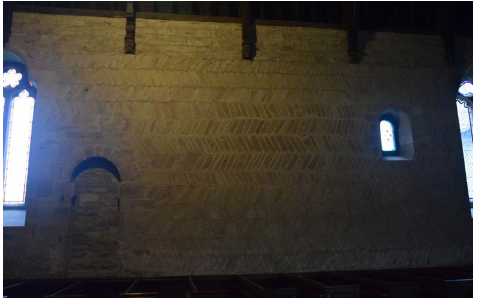
Distinctive herringbone pattern in the north wall of St Peter's Church in Diddlebury
