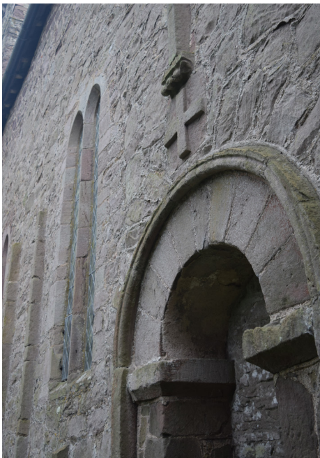
Detail of the north door where the Romanesque arch has been framed by characteristic Saxon moulding
